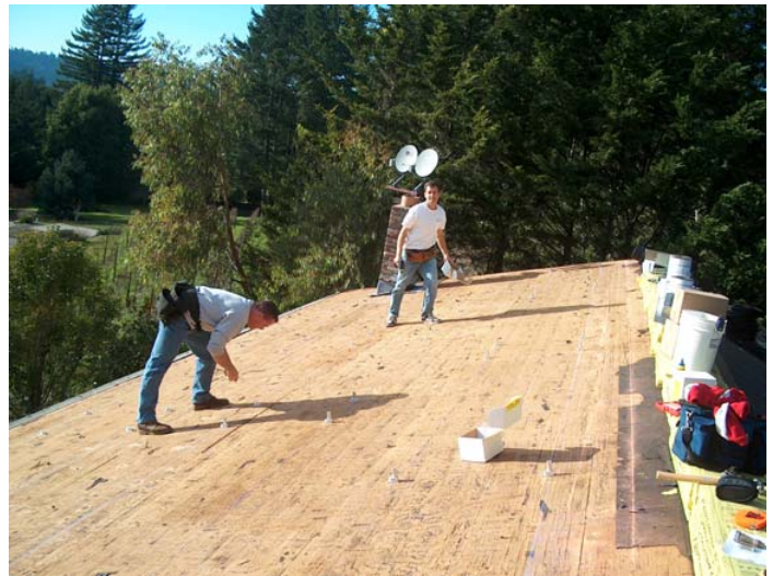
The Keiths prepare the roof of a home for solar panel installation
